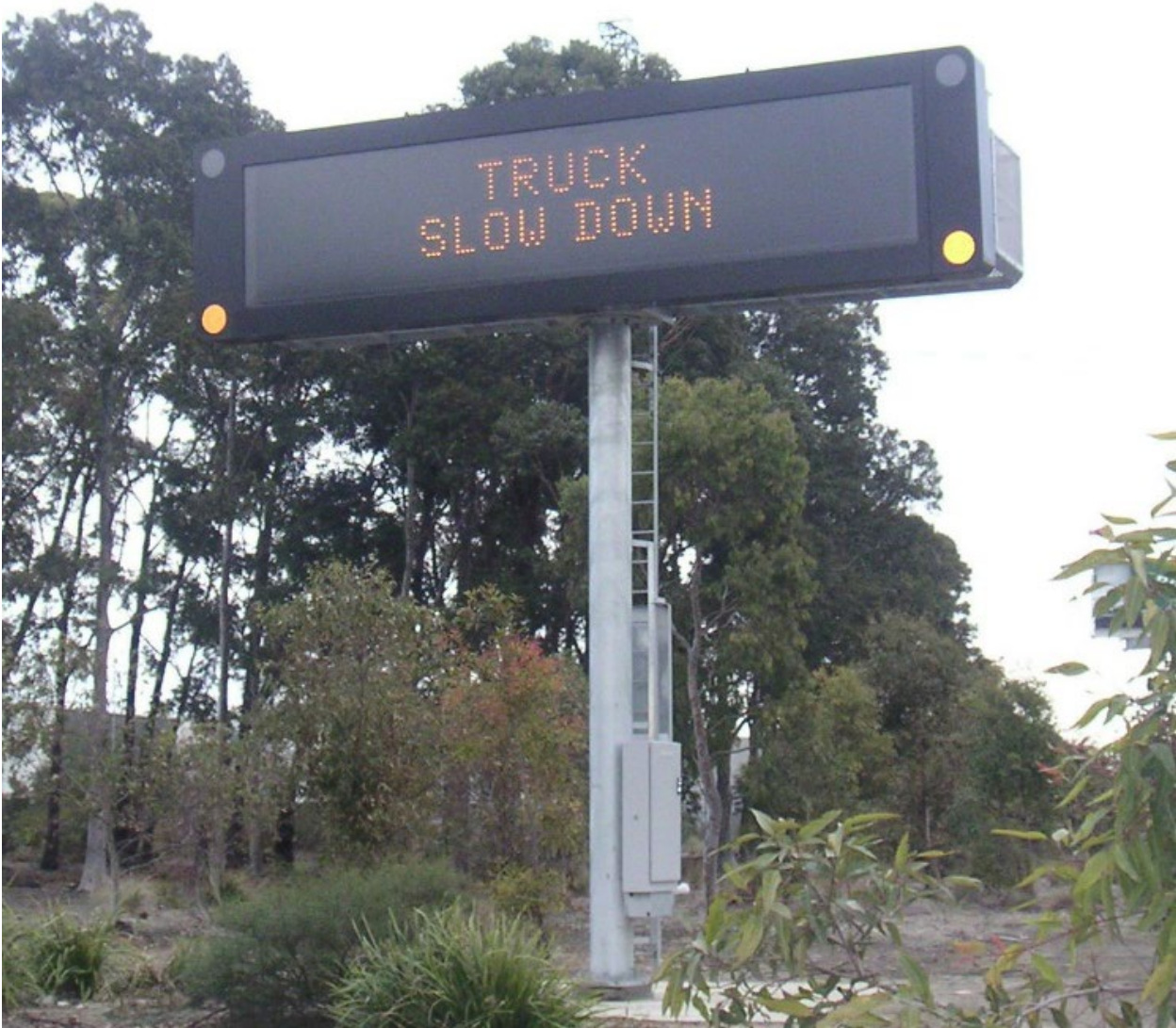
Figure 5.11: Vehicle activated warning sign for trucks
